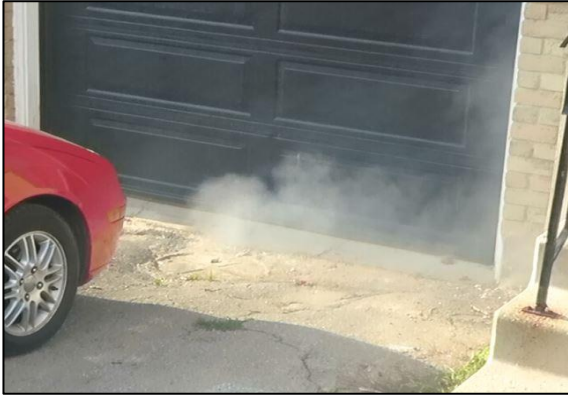
Smoke at reverse-sloped driveway CB indicating a direct connection with storm sewer.
