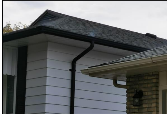
Smoke out of downspout indicating a direct connection with storm sewer.
