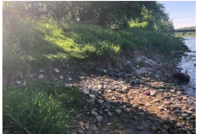
Photograph 6: Bank erosion on left downstream bank just downstream from Brant's Crossing Bridge.
