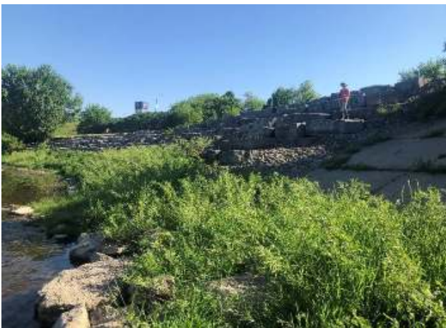
Photograph 9: Riprap along left downstream bank on upstream side of Brant's Crossing Bridge.
