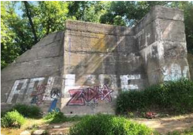
Photograph 5: Old bridge abutment on left downstream bank just downstream from TH&B Rail Bridge.
