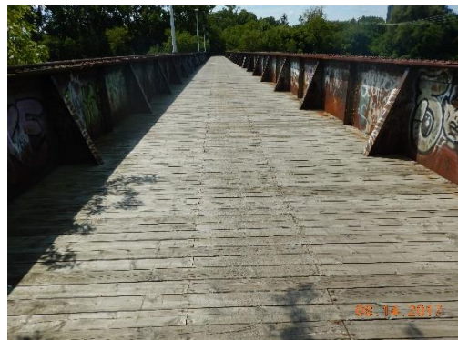
Figure 8: TH&B Crossing Bridge deck top (no deck drains present)
