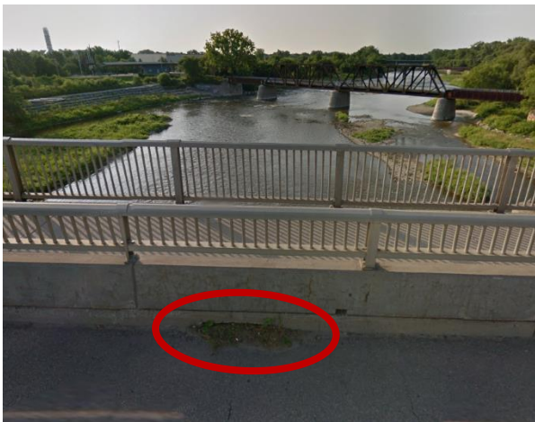
Figure 1: Southern deck drain inlet at center arch, clogged with debris
