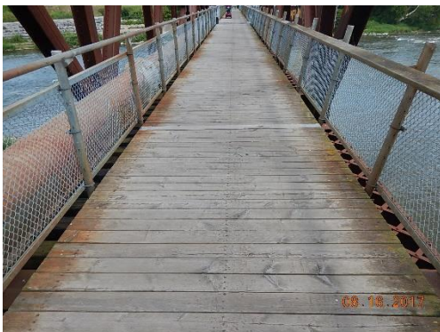
Figure 7: Brant's Crossing Bridge deck (no deck drains present)
