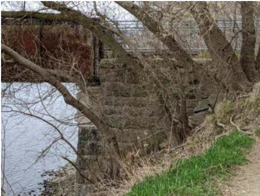
Figure 64: View facing north of the east abutment of the TH&B Crossing Bridge
