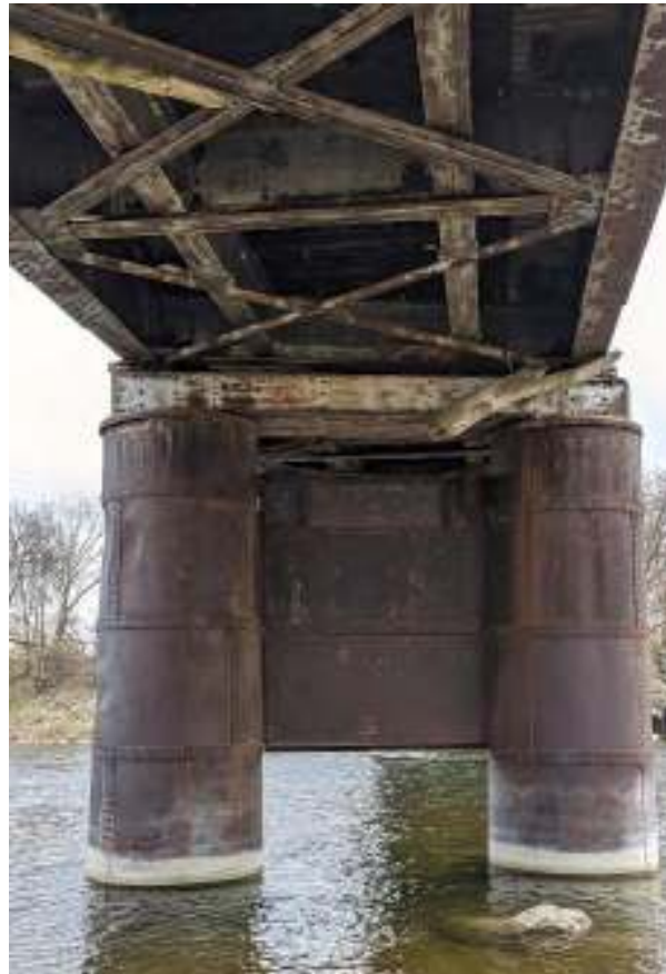
Figure 70: Capping beam over the central pier bent, which supports the girder composed of bottom flange plates and stringers linked by transverse beams or cross girders on gusset plates, all with lateral cross bracing.
