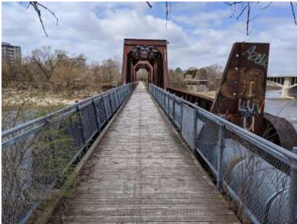
Figure 53: Decking and utility corridor (with metal access barrier) at the east approach
