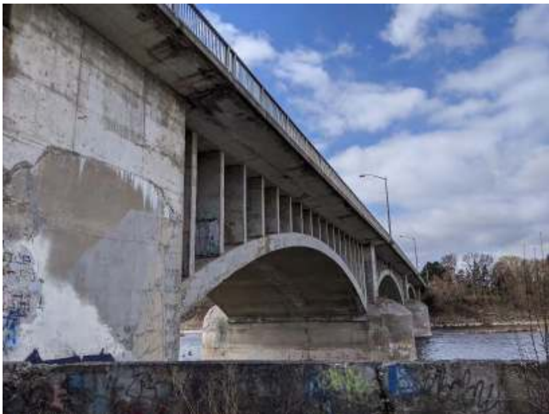
Figure 21: View west from the east abutment of the solid and thin concrete slab deck with chamfered soffit
