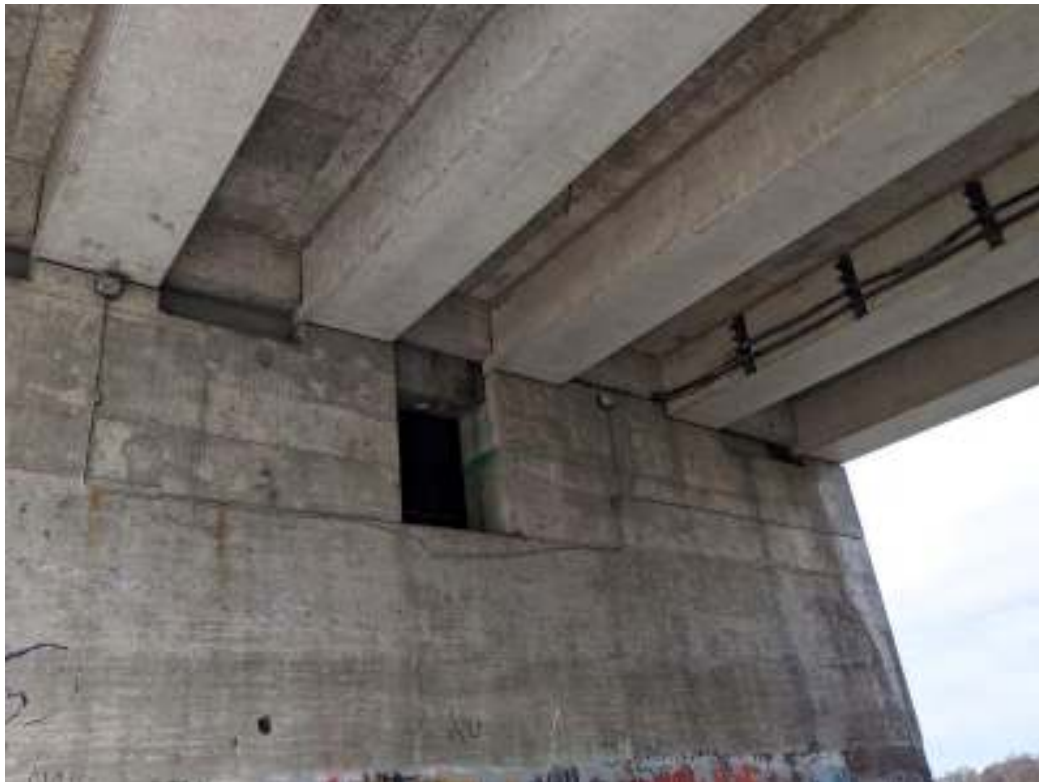
Figure 14: Narrow crenulated bearing shelf on the east side of Lorne Bridge east abutment, where it supports the girder of the Lorne Bridge Girder Span
