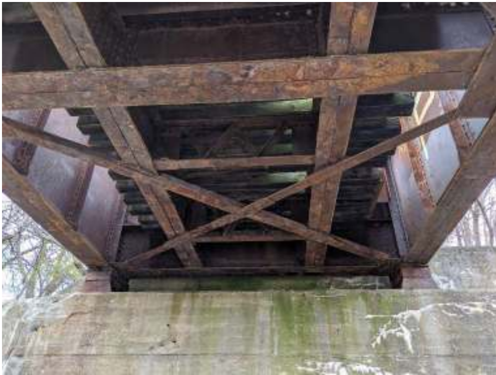
Figure 42: Construction visible on the underside of the west girder including the fixed bearings, transverse beams or cross girders on gusset plates, and lateral cross bracing. Above this can be seen the two stringers with transverse beams and short intermediate lattice trusses, which are capped by closely spaced wood ties.
