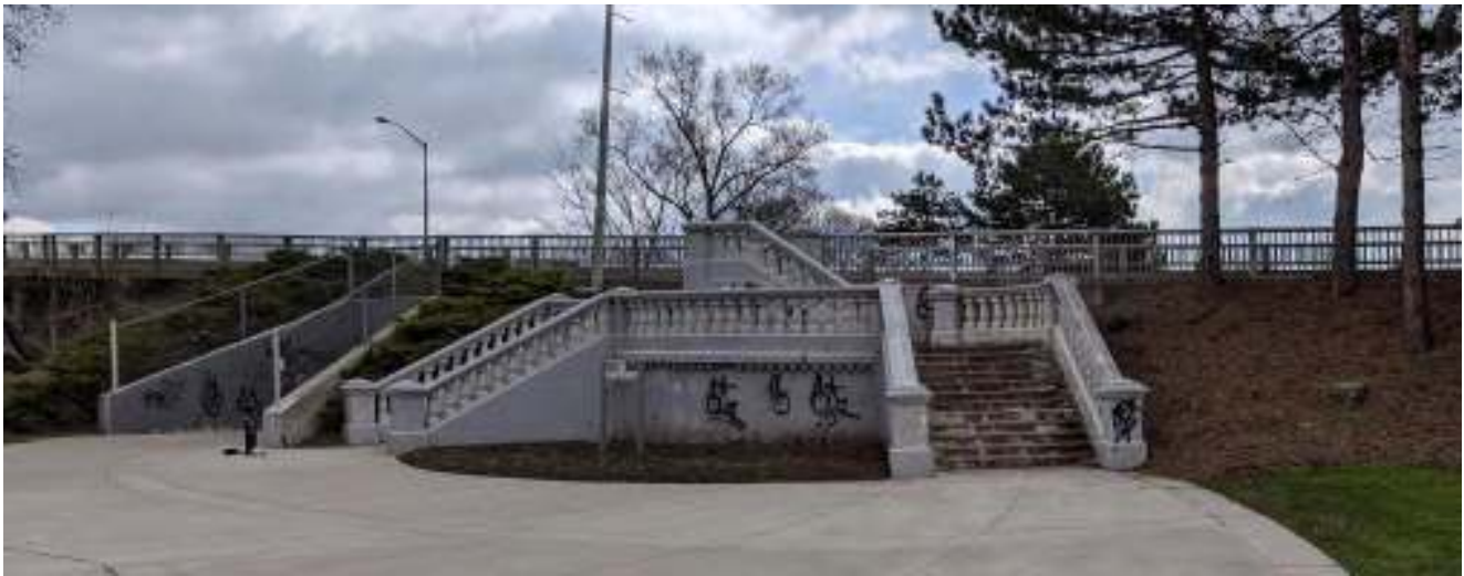
Figure 24: Bifurcated concrete stairs on the north side of the west approach, facing south from Lorne Park
