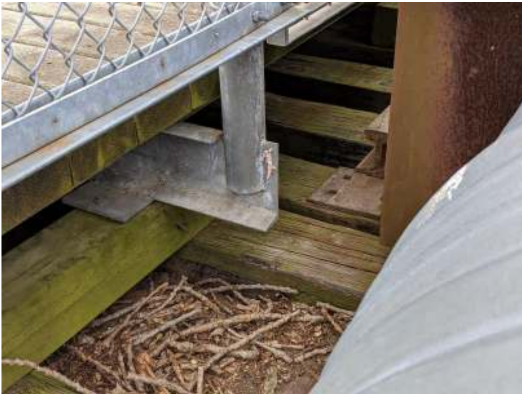
Figure 44: Remnants of the rail track (centre right) on the deck of the west approach span
