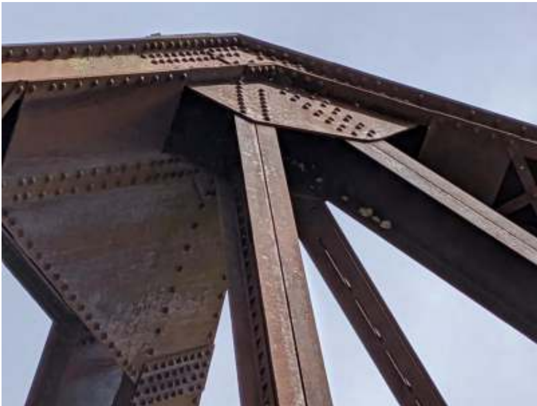
Figure 48: Detail of the end post of the west span showing the connection with the top chord, sway bracing, vertical post and diagonal and plating at the portal
