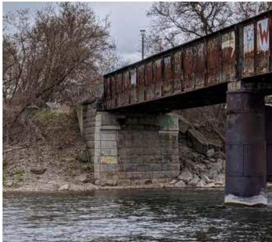
Figure 66: View facing southeast of the east abutment with ashlar construction and concrete repairs
