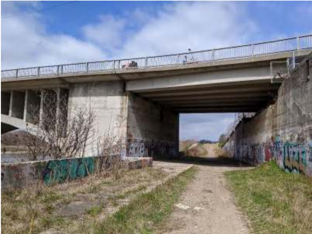
Figure 13: The Lorne Bridge Girder Span that forms the east approach of the Lorne Bridge
