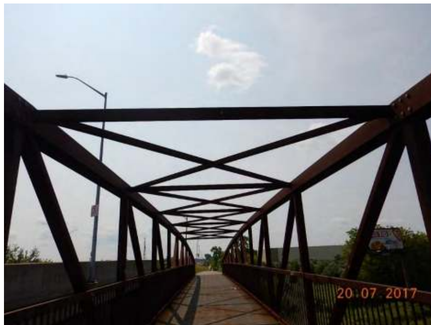
Figure 77: View from the deck of an example of a prefabricated steel through truss pedestrian bridge (courtesy GM BluePlan)
