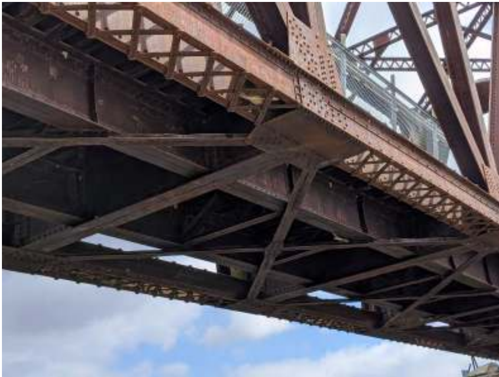
Figure 50: Detail of the west span construction showing the bottom chord with crossed lateral bracing, stringers with short intermediate trusses and lateral cross bracing on gusset plates
