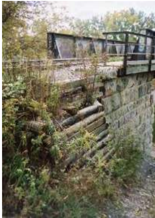
Figure 65: Wood cribbing at the east approach (Photo by Charles Cooper, Collection of Brant Railway Heritage Society)
