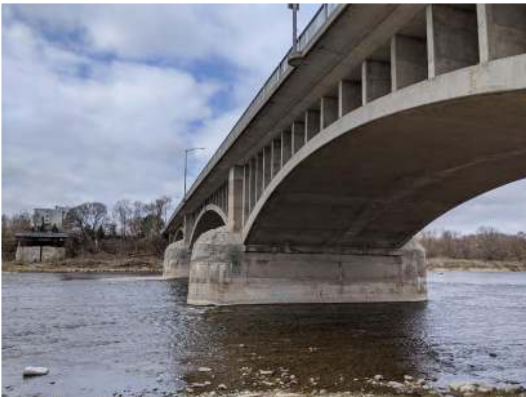
Figure 16: View west of the downriver sides of Pier No. 1 and Pier No. 2
