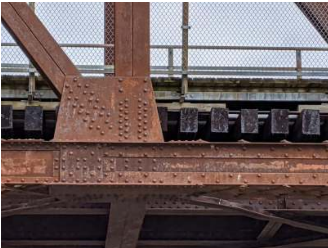
Figure 49: Gusset plates at the diagonal and vertical post, and the wood ties of the deck
