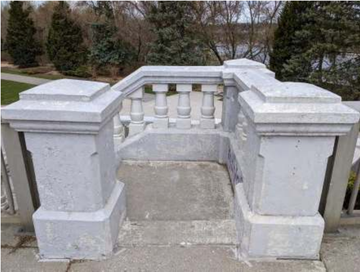
Figure 26: Half-pace landing at the west approach deck with thick square newels with chamfered and moulded caps, chamfered corners, and thick pedestals
