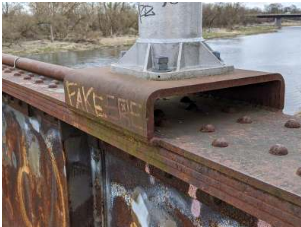
Figure 75: Conduit and aluminium light standard mounts on the top flange plate
