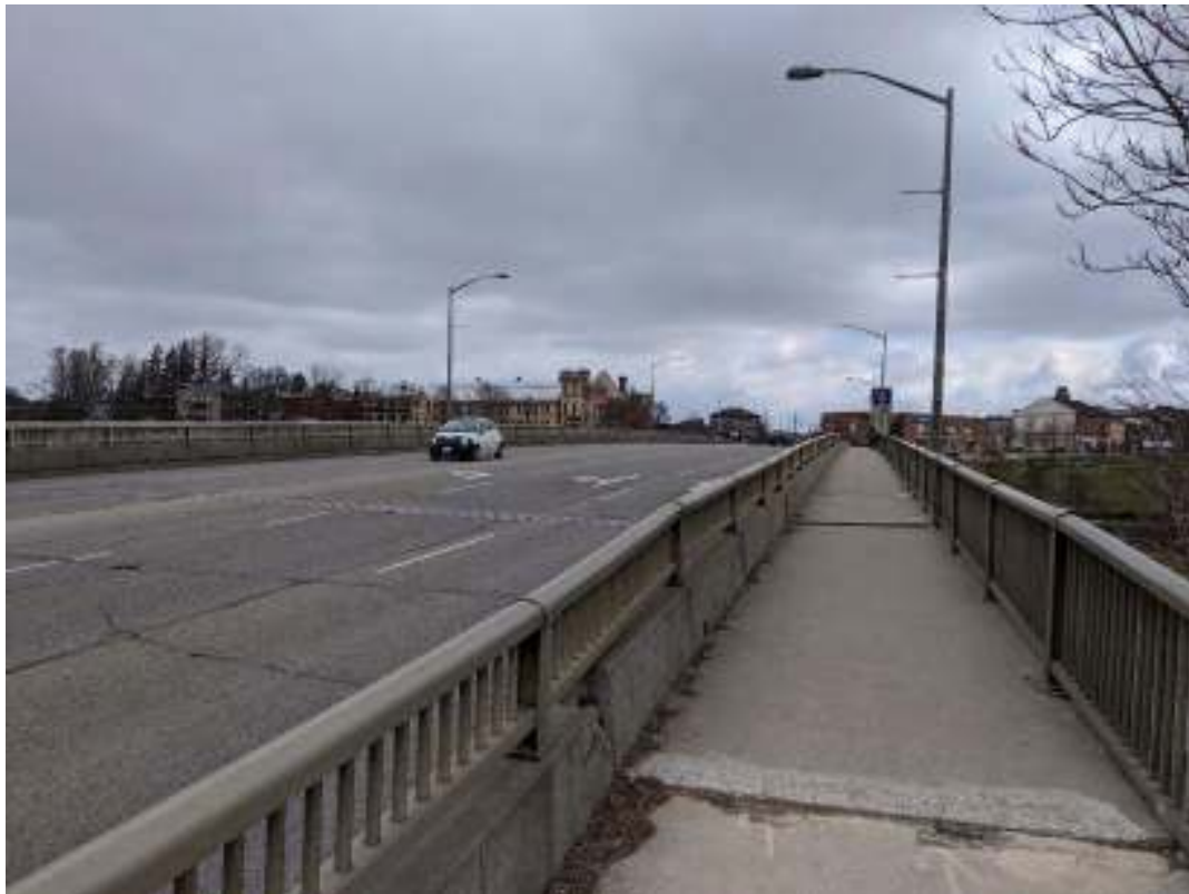
Figure 22: View east from near the centre of the bridge of the deck camber from the east and west, low cast-in-place concrete parapet walls with single railings either side of the asphalt wearing surface, and cast-in-place concrete sidewalk with aluminium post and panel railings
