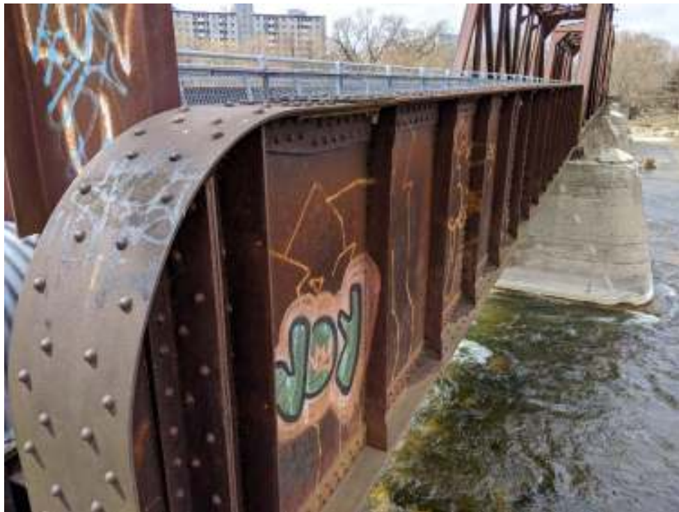
Figure 43: Riveted girder web plates with vertical stiffeners on the east approach span
