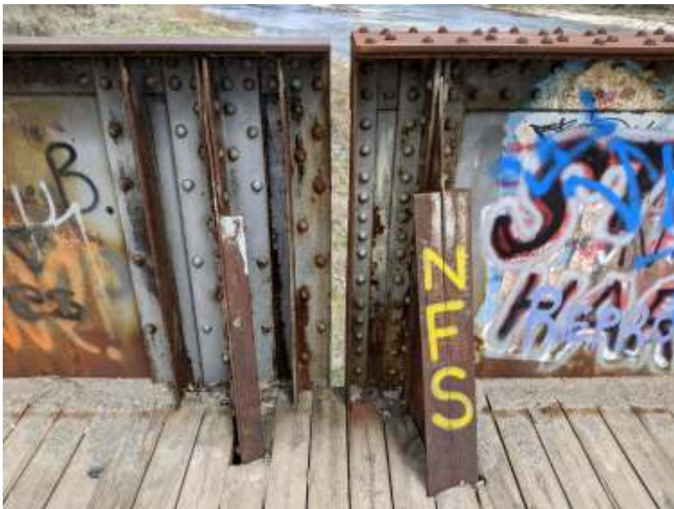
Figure 74: Joint between the west approach span and centre west span showing varying construction
