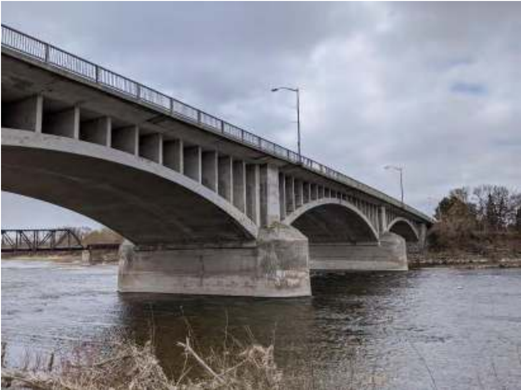
Figure 17: View west of the upriver sides of Pier No. 1 and Pier No. 2
