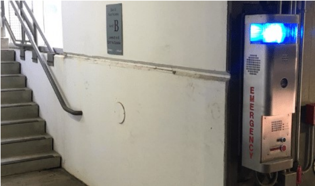
Figure 28 - Example of Emergency Call Station
