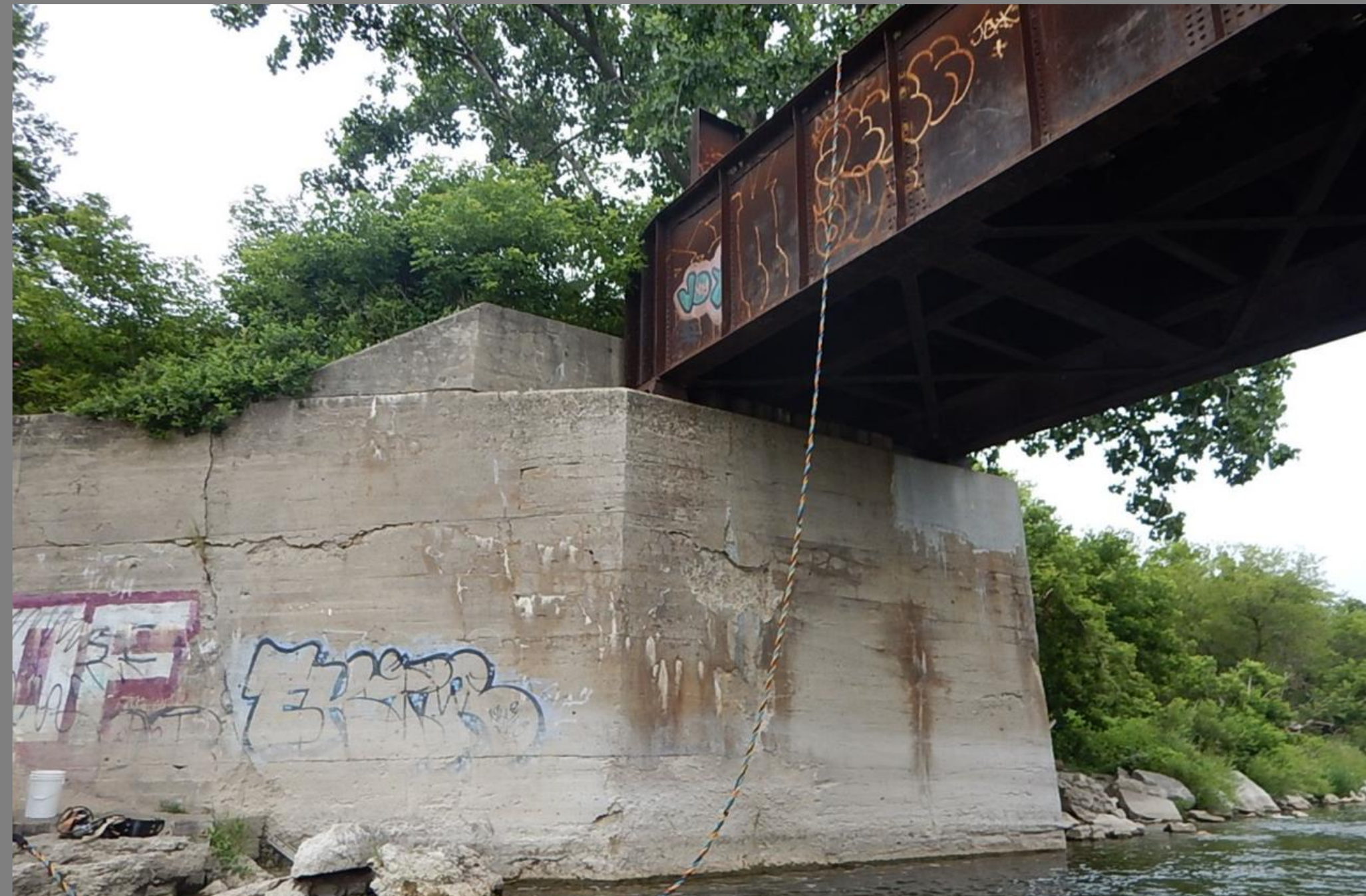
Deterioration of concrete abutment
