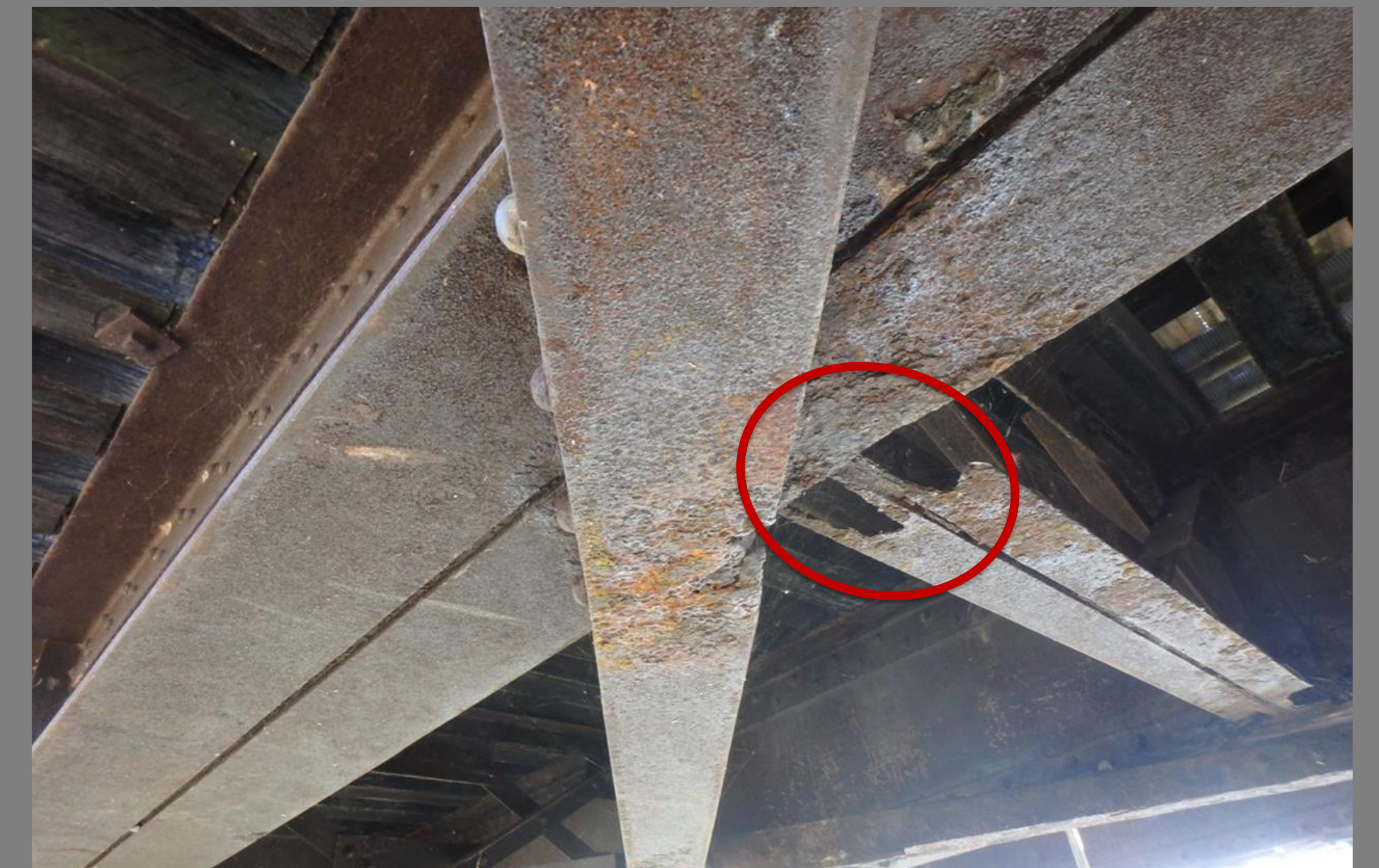
Section loss on diaphragms
