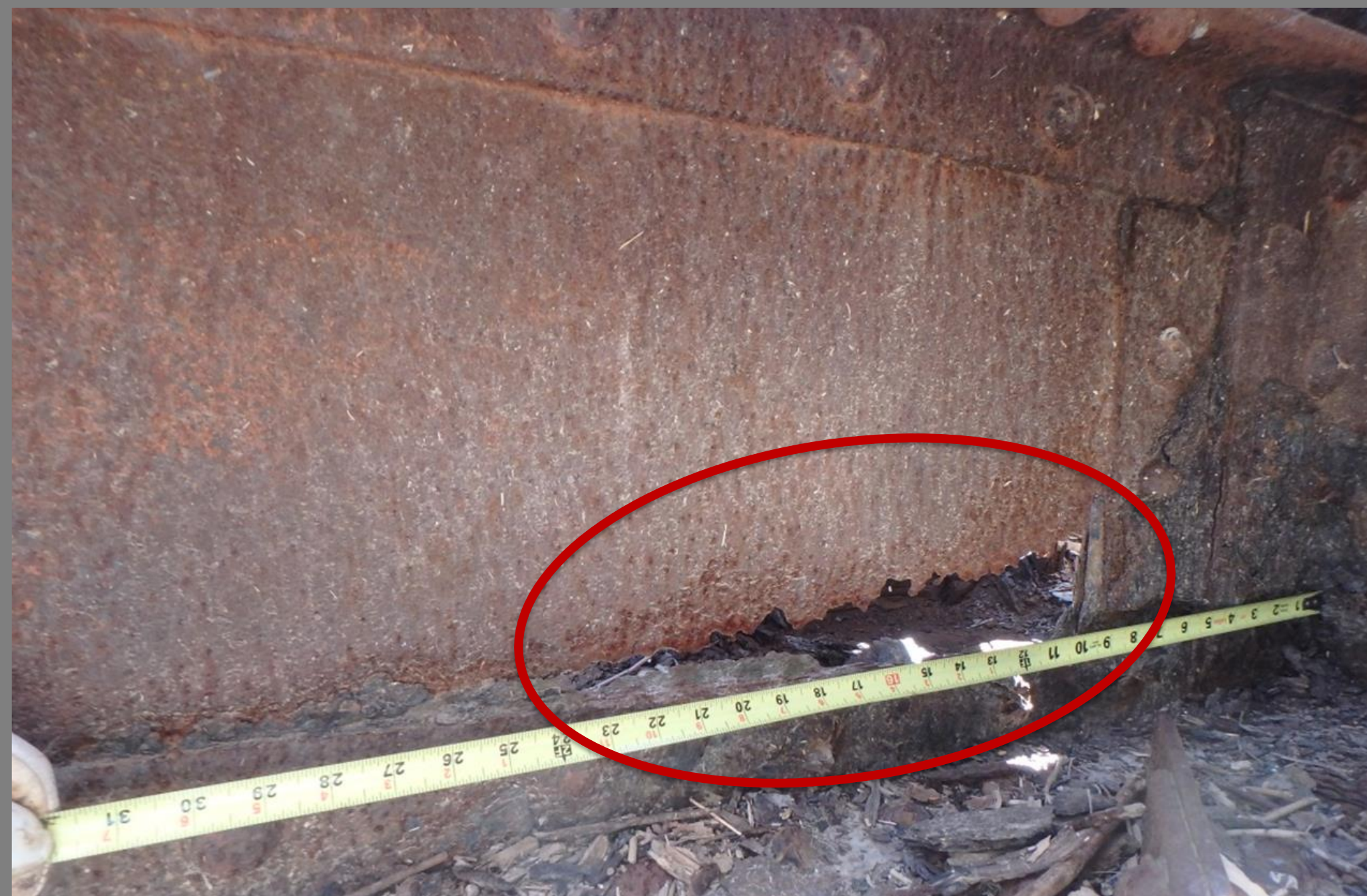
Complete loss of section on floor beams
