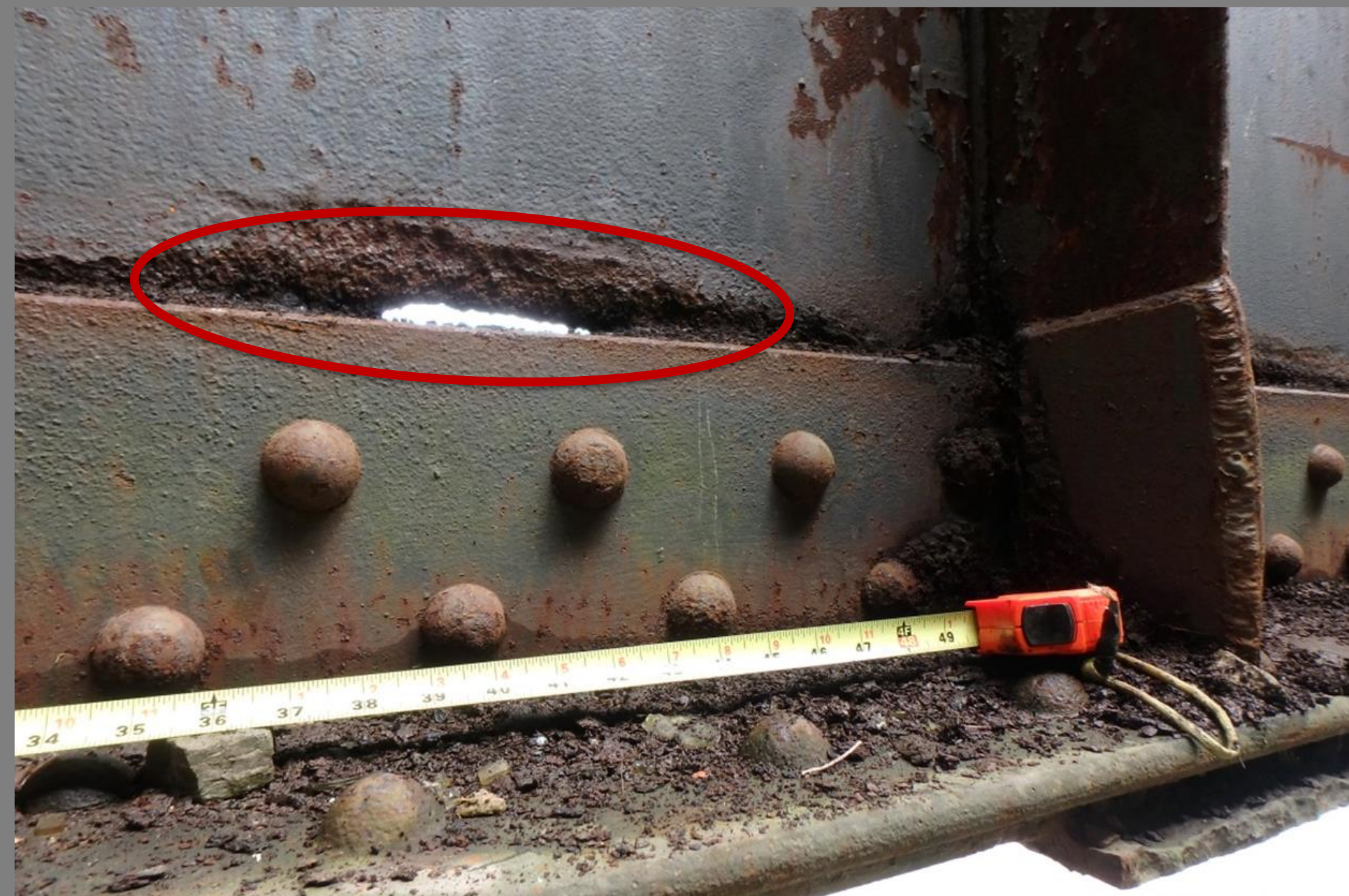
Complete loss of section on girders
