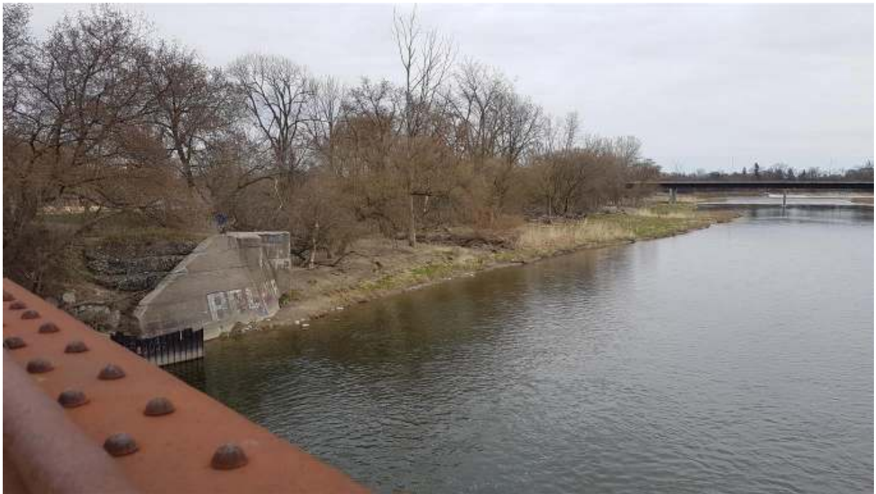
Image 6: Concrete bridge pier of the former Lake Erie and Northern Railway within the Study Area; facing east, April 24, 2020.
