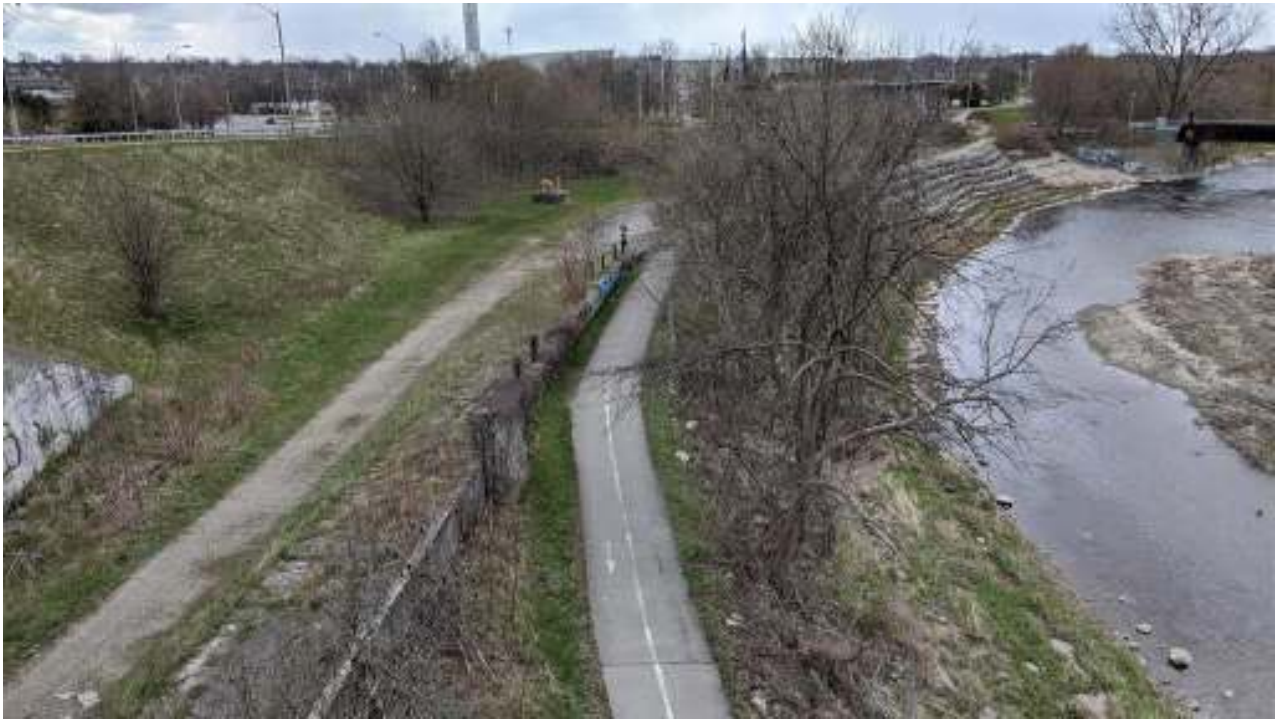
Image 7: A representative example of the City of Brantford's dike system; facing southeast, April 24, 2020.
