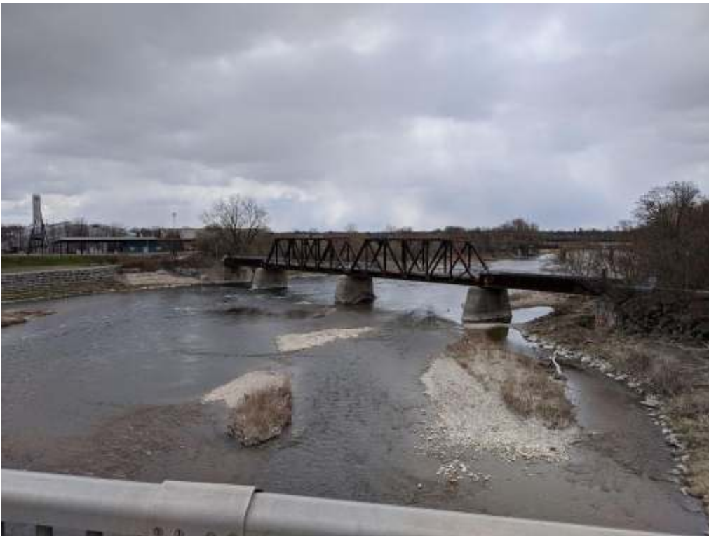
Photograph 9: View of the Brant's bridge from the Lorne bridge to the south, facing northeast.
