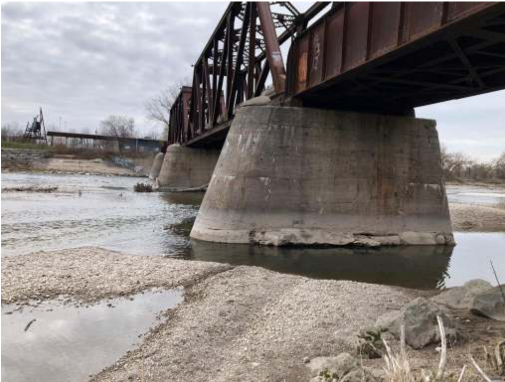
Photograph 10: Brant's bridge- Looking at west pier from the upstream side of the bridge and west abutment.
