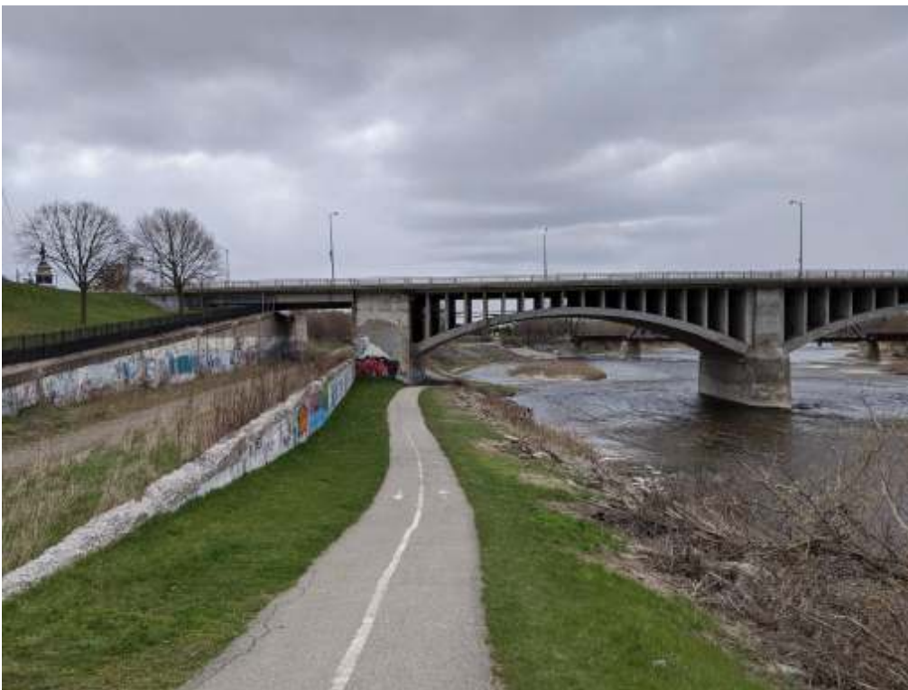
Photograph 5: Lorne bridge – Looking at east pier and abutment from upstream side of the bridge.
