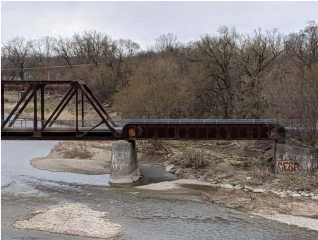
Photograph 13: Brants bridge – Looking at west pier and west abutment from upstream side.
