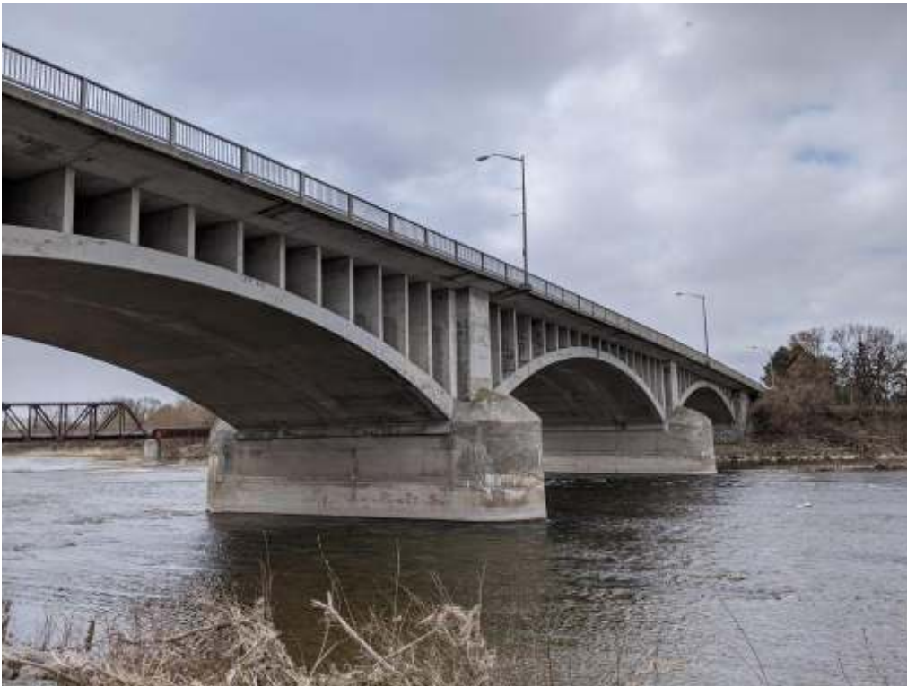
Photograph 6: Lorne bridge – Looking at east pier and west pier from upstream side of the bridge.
