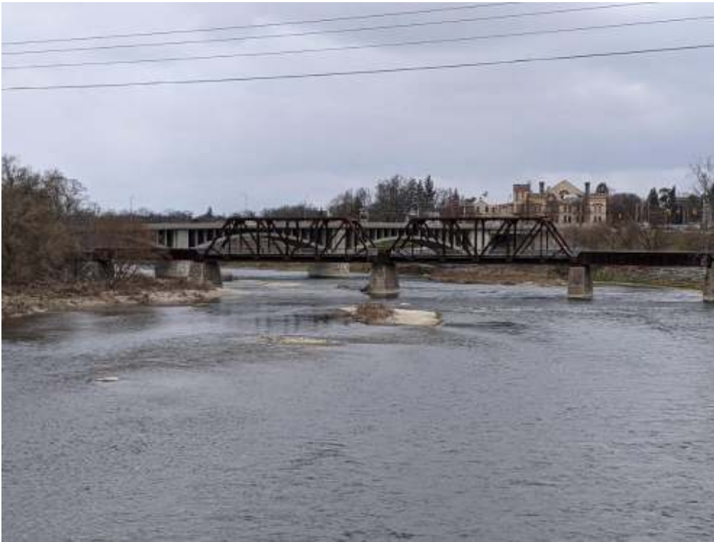
Photograph 4: View of the Brant's and Lorne bridge from the TH&B Crossing Bridge to the south, facing north.
