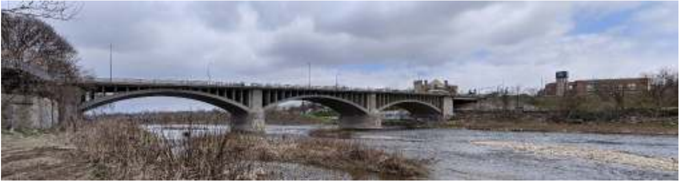
Photograph 1: View up-river to Lorne Bridge and downtown Brantford from the west abutment, facing north.
