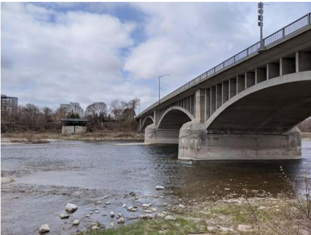
Photograph 7: Lorne bridge – Looking at east pier and west pier from downstream side.
