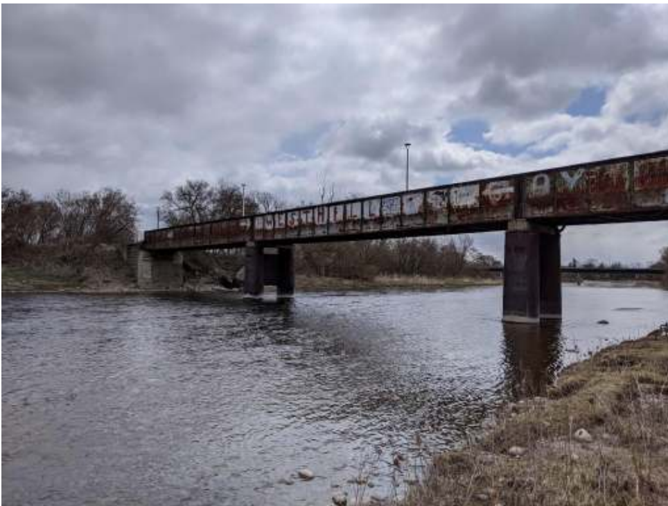
Photograph 15: TH&B Crossing Bridge – Looking at central pier, east pier and east abutment from upstream side.
