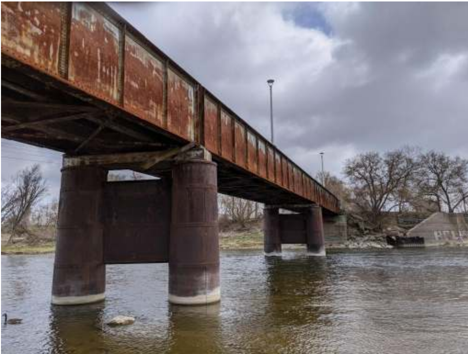
Photograph 14: TH&B Crossing Bridge– Looking at central pier, east pier, and east abutment from downstream side.
