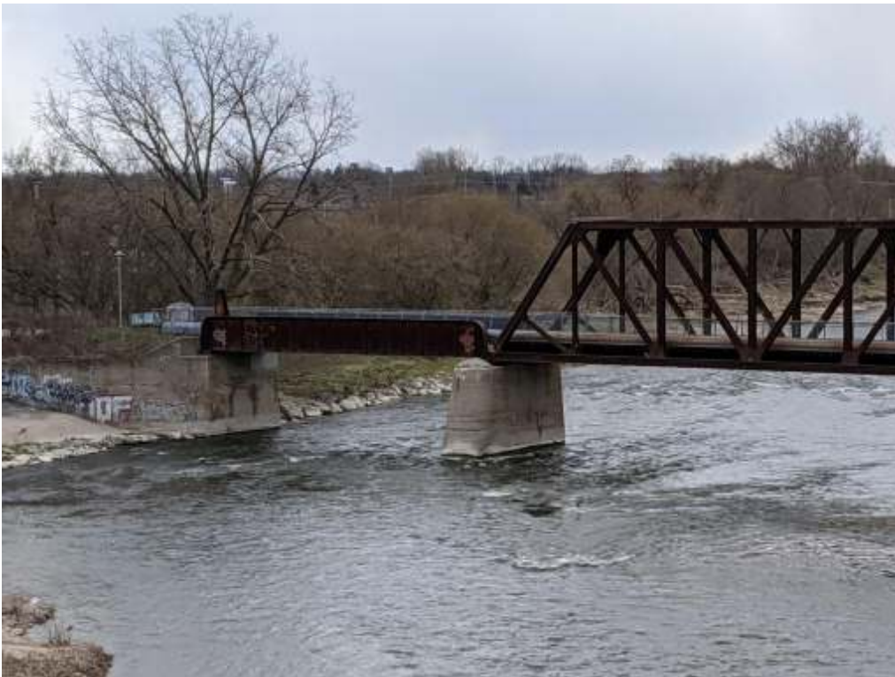
Photograph 11: Brant's bridge- Looking at east pier and east abutment from upstream side.
