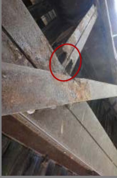
Section loss on diaphragms
