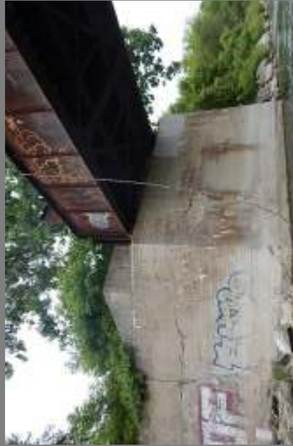
Deterioration of concrete abutment
