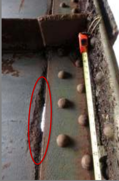
Complete loss of section on girders
