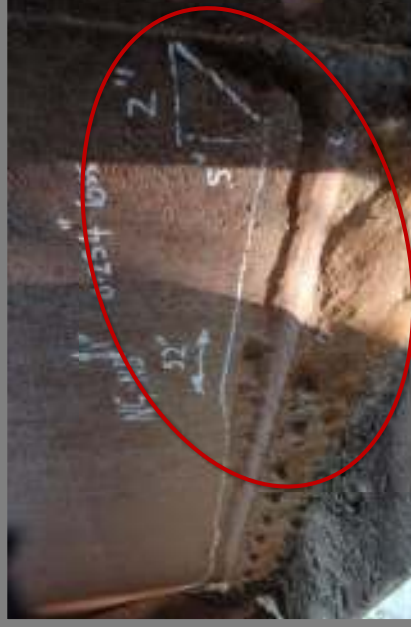
Severe corrosion on girders
