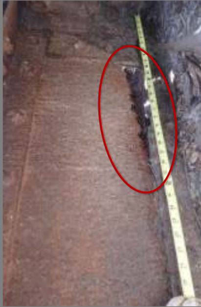
Complete loss of section on floor beams
