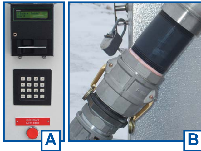
A. Fill Station Key Pad. B. Fill Station Attachment Couplings
