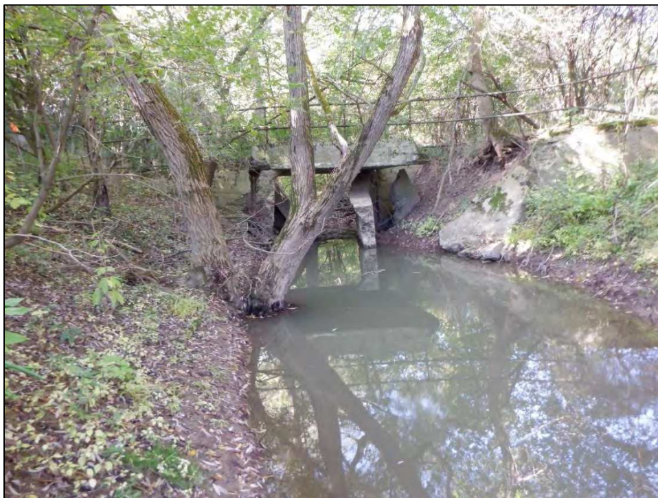
Figure 3.84: Channel Incision at Reach LF Trib B
